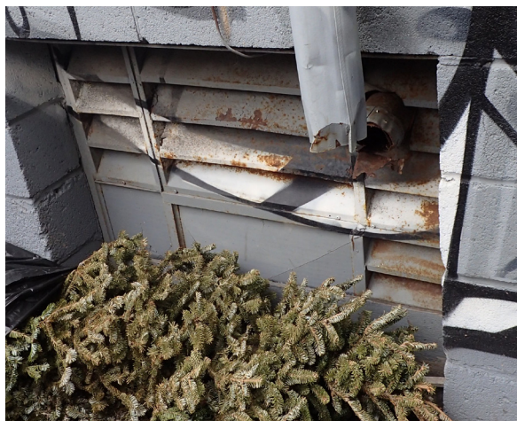
65. Rusting louvered vent, North elevation.
