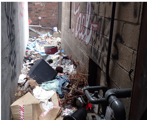
59. Garbage blocking alley at West elevation.
