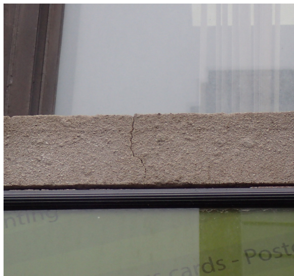
46. Crack in window sill, South elevation.
