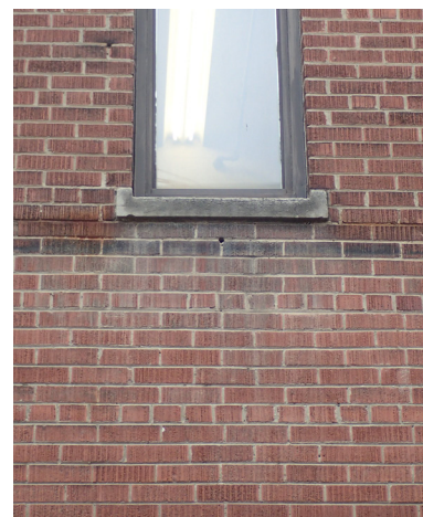
44. Staining to masonry underneath window sill, South elevation.
