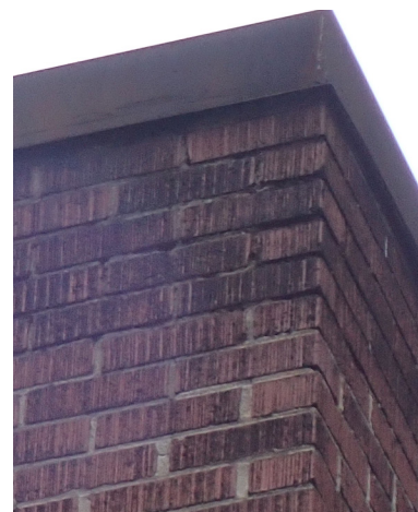
43. Open mortar joints in upper courses at roof level, South elevation.
