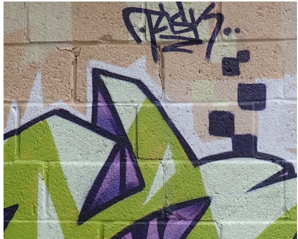
70. Stepped crack through concrete block work and mortar joints, East elevation.
