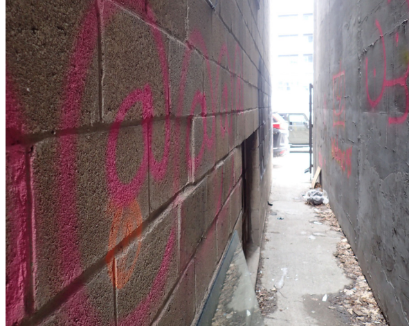
56. Concrete block work not plumb, West elevation.
