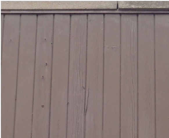
51. Example of wooden panels splitting, South elevation.
