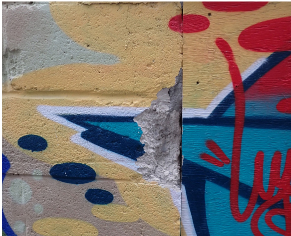
69. Chipped concrete block, East elevation.
