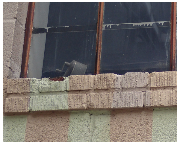
66. Spalled brick in brick sill, East elevation.
