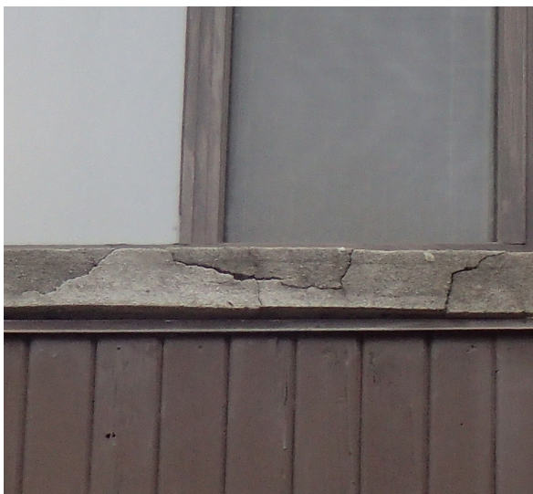
47. Defective window sill with multiple cracks, South elevation.
