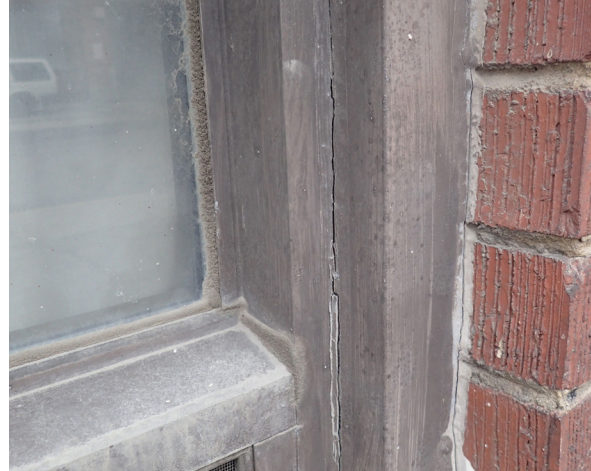
50. Example of cracking and separating sealant at windows, South elevation.
