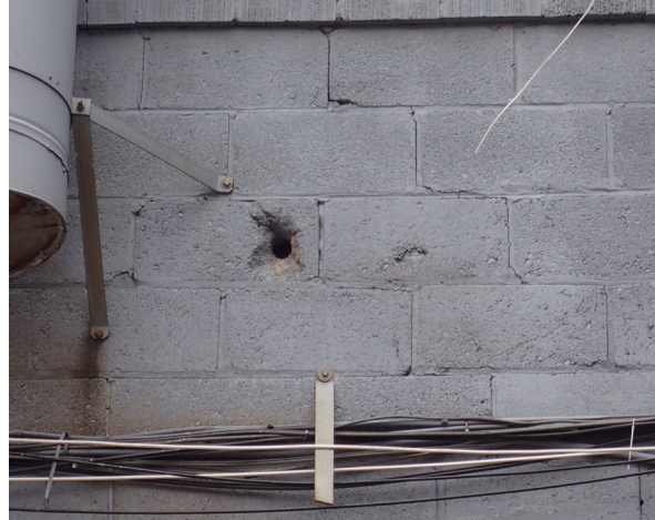
62. Example of hole in block work, North elevation.
