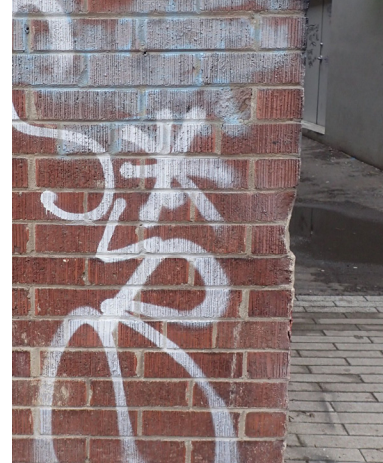
42. Graffiti staining to bricks, and chips to bricks, South elevation.
