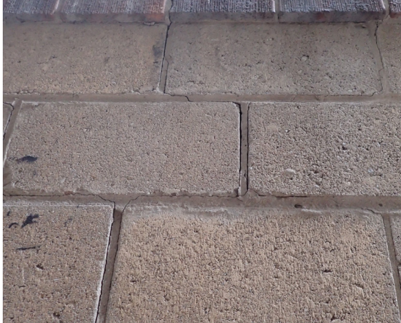
55. Stepped crack through mortar joints, West elevation.
