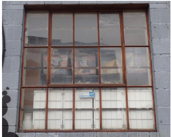
64. Rusting of steel windows, North elevation.
