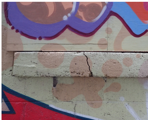
71. Crack in concrete sill, East elevation.
