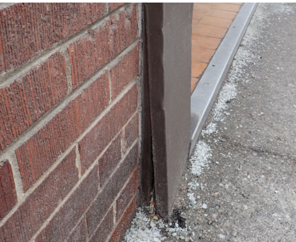
53. Damaged base of metal frame at recessed entrance, South elevation.
