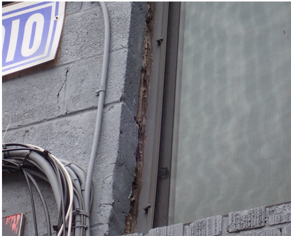
63. Poor condition of caulking at aluminium window, North elevation.
