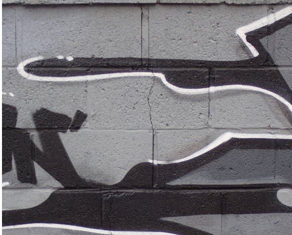
61. Example of cracks through mortar joints and block work, North elevation.
