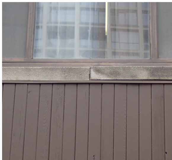
48. Example of open mortar joints in window sill, South elevation.
