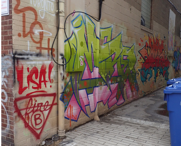
67. Painted block work, and graffiti staining, East elevation.
