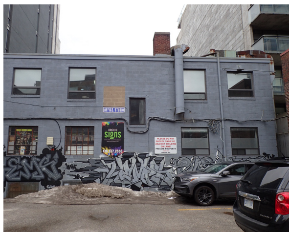
60. Painted block work with graffiti staining, North elevation.
