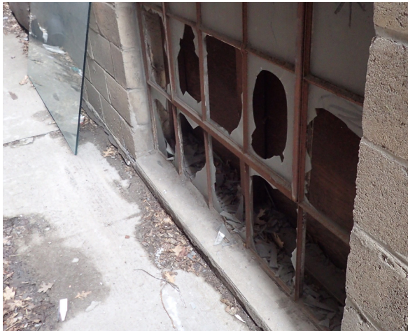
57. Broken glass in steel window, West elevation.
