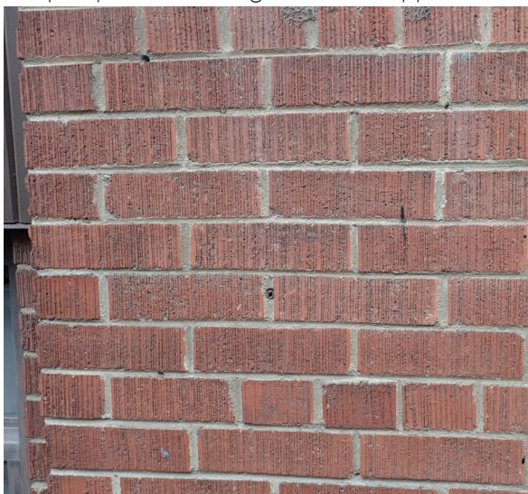
45. Example of good condition of bricks and mortar joints. Note plugs left in mortar, South elevation.
